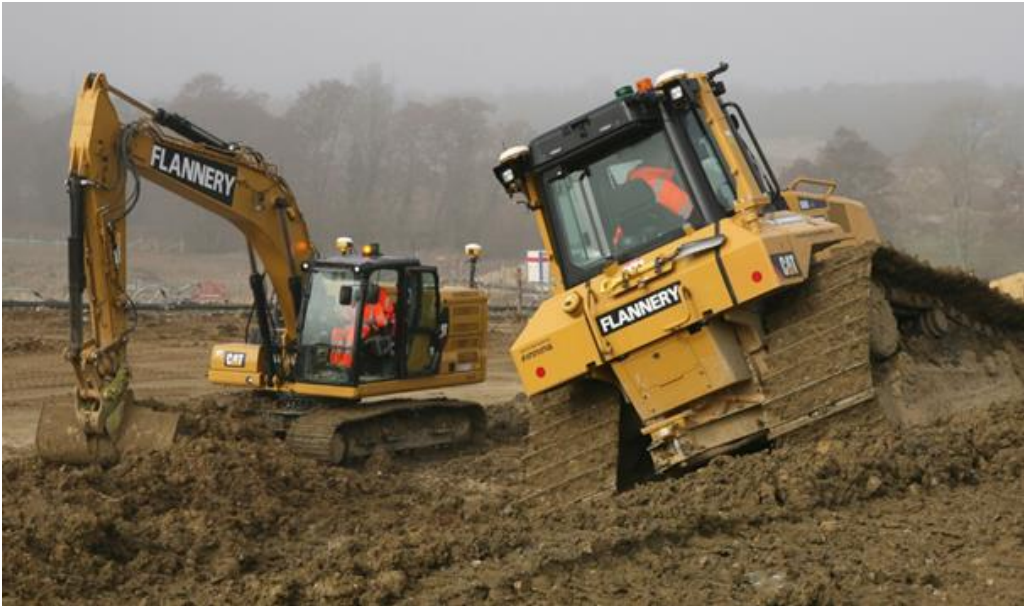
Figure 23 – CAP retrofitted enabled plant in operation
