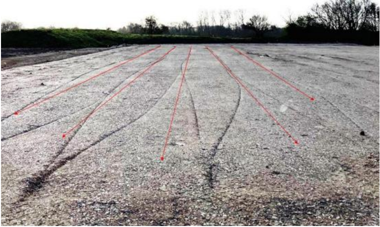
Figure 21 - Manual compaction showing misalignment of passes and overlaps.
