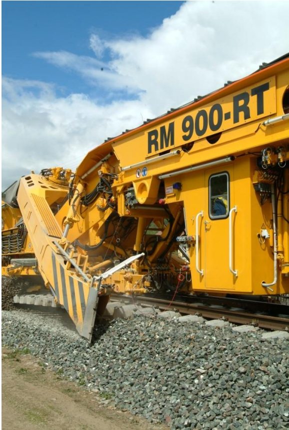
Figure 7 - Network Rail's ballast cleaner system (BCS) in operation, which limits worker exposure to hazards xxvi
